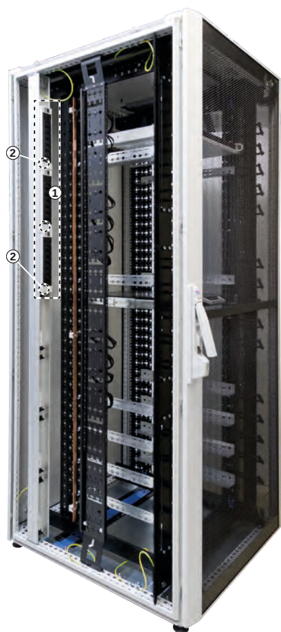
Fig. 6: Power distribution bar ① mounted on the left-hand traverse
