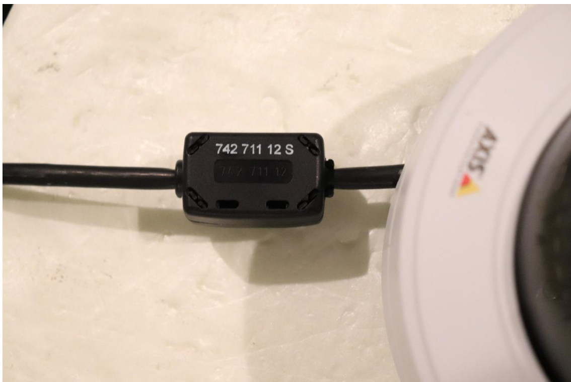
Photograph 6. Added ferrite core on the baseline camera cable
