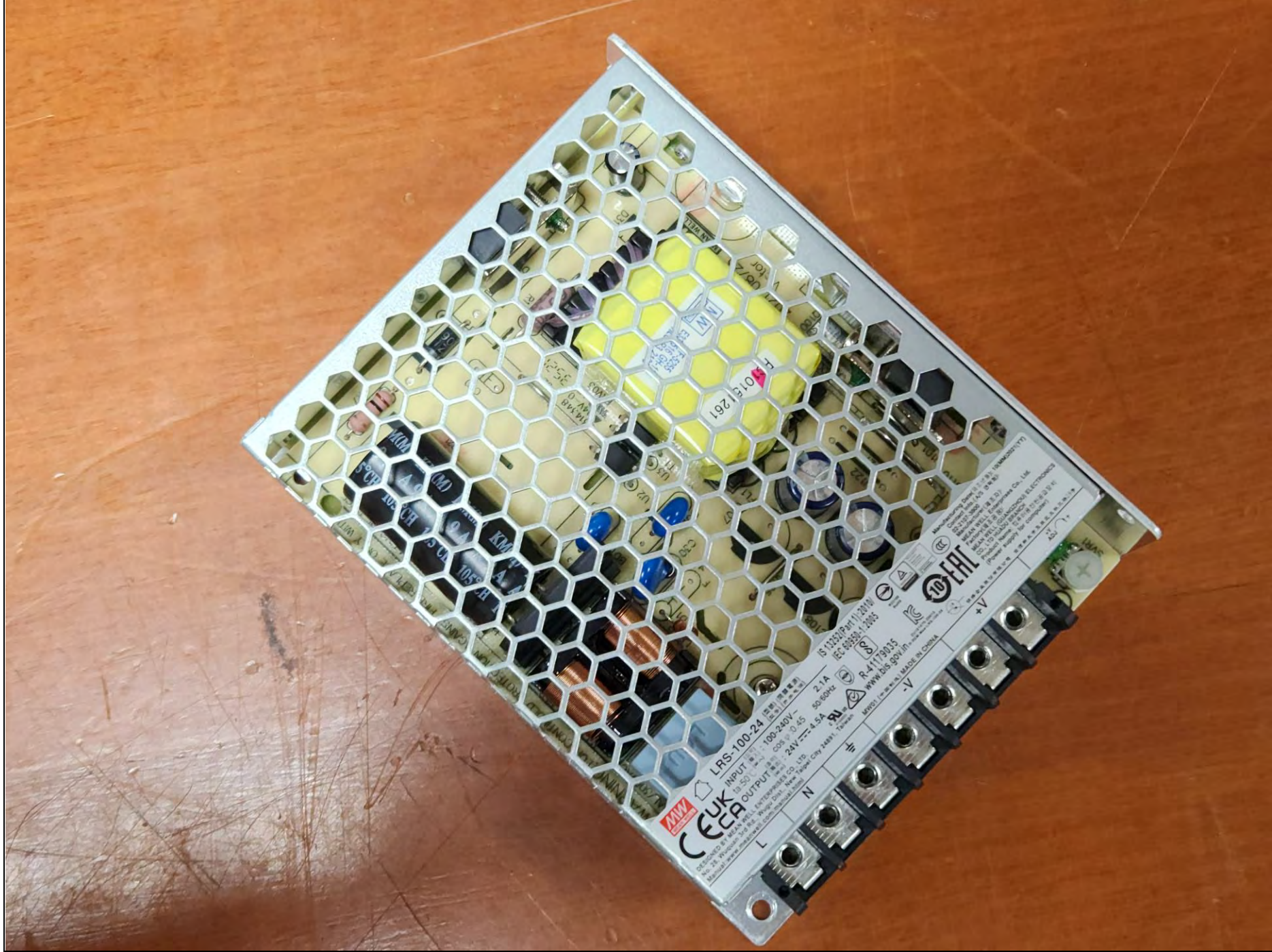
Front View of Controller SMPS2
