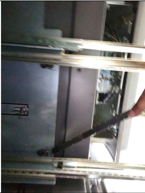
8. Cable way inside ATM
