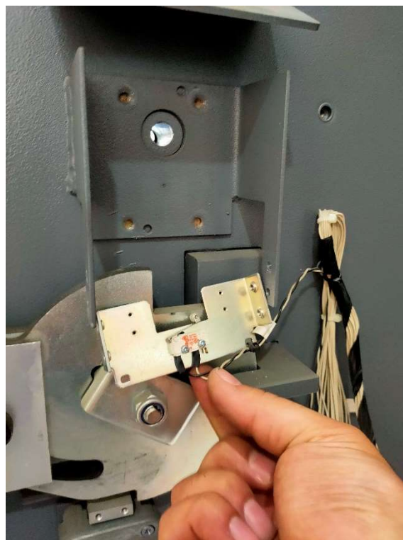
8. It is not mandatory to use this piece of metal for future installation
