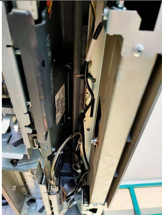
2. Already existing cables on the front door
